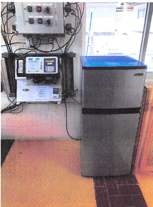
Current Retrofitted Sampler
