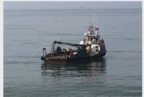
Picture above: Harbor Offshore's boat is on location. Divers are installing the repair clamp on the outfall pipe.
